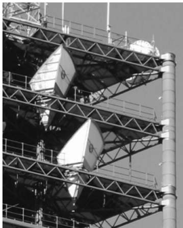
Figure 4-14 Telephone transmission tower showing two horn antennas
